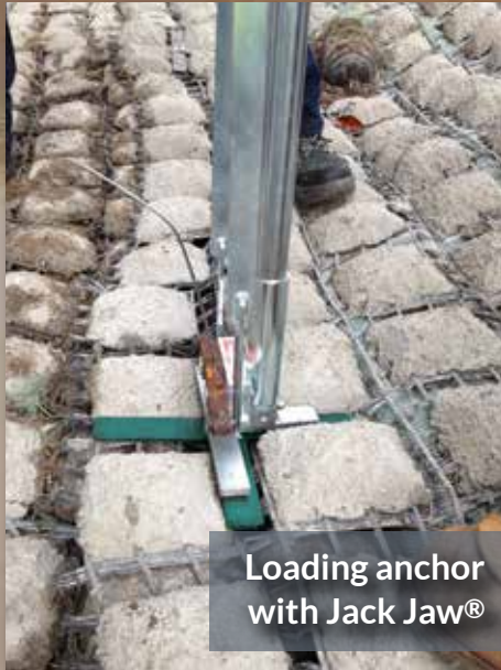
Gas powered driver installation
